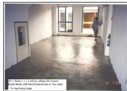
W1 + cement to prevent rising dampness Pasir Panjang Village. 2010 June
