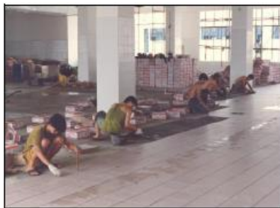
Tiling work by using W1 cement mortar Camel Nut Factory, Defu Lane 10. 2010 August
